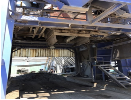
<Ascon mixing machine>
